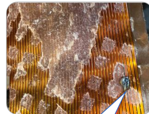
Winding to Winding failure with Kraft paper removed from Layer, exposing individual windings
