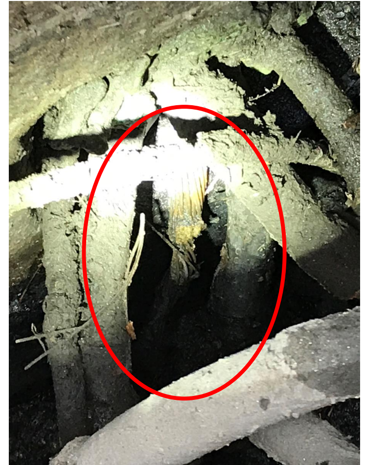
Neutral broken/corroded in the service box
