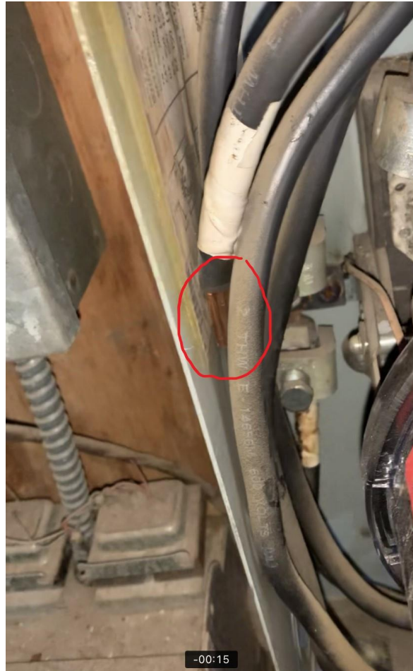
Neutral not connected in the meter pan
